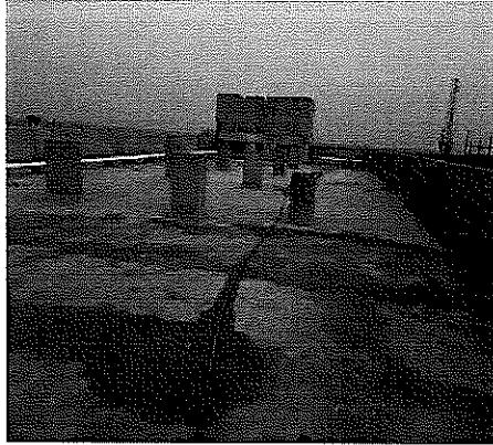
WATERPROOFING AT ROOF LEVEL COMPLETED ALONG WITH CONSTRUCTION OF OVERHEAD WATER STORAGE TANK
