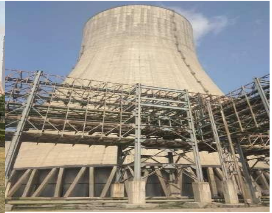
A photograph of cooling tower installed in PPGCL
