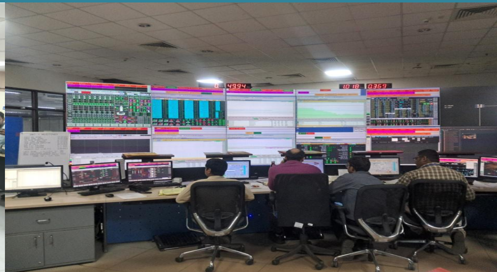
A monitoring of power generation and grid (demand/supply) at Meja Thermal Power Station, Meja, Prayagraj, Uttar Pradesh.
