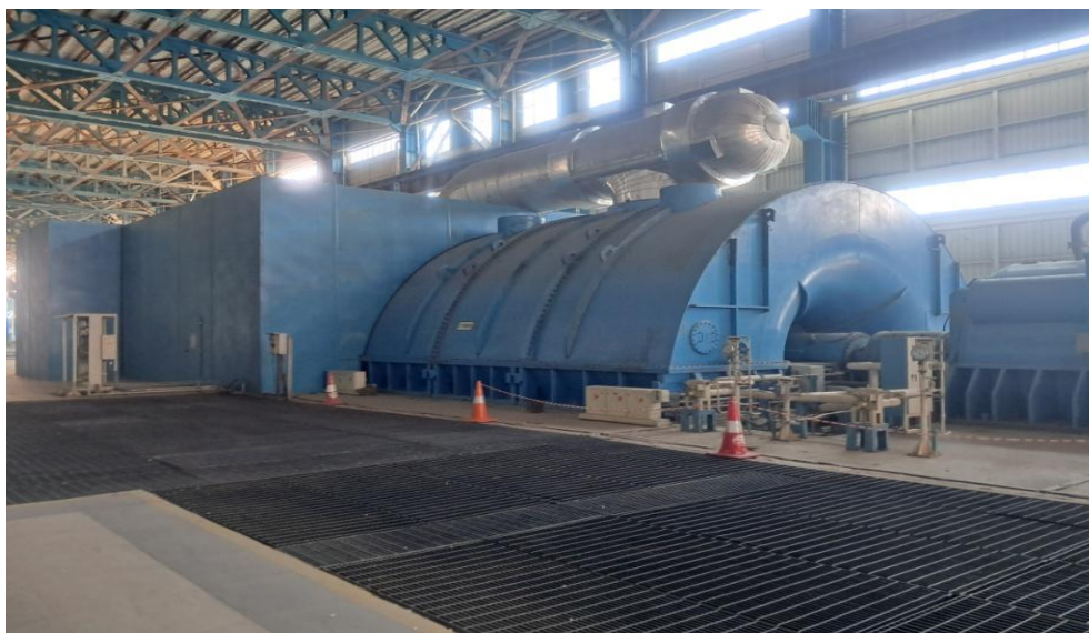
A photograph of turbine and generator assembly at Meja Thermal Power Station, Meja, Prayagraj, Uttar Pradesh
