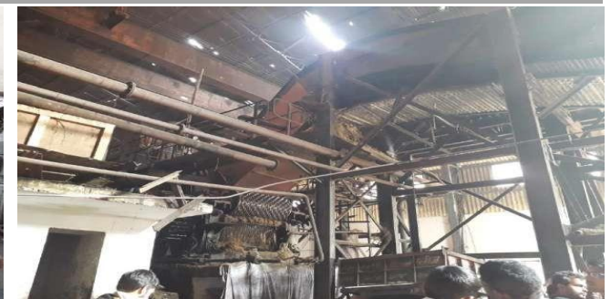
A photograph of steam turbine with generator installed for power generation at KSCML, Sultanpur
