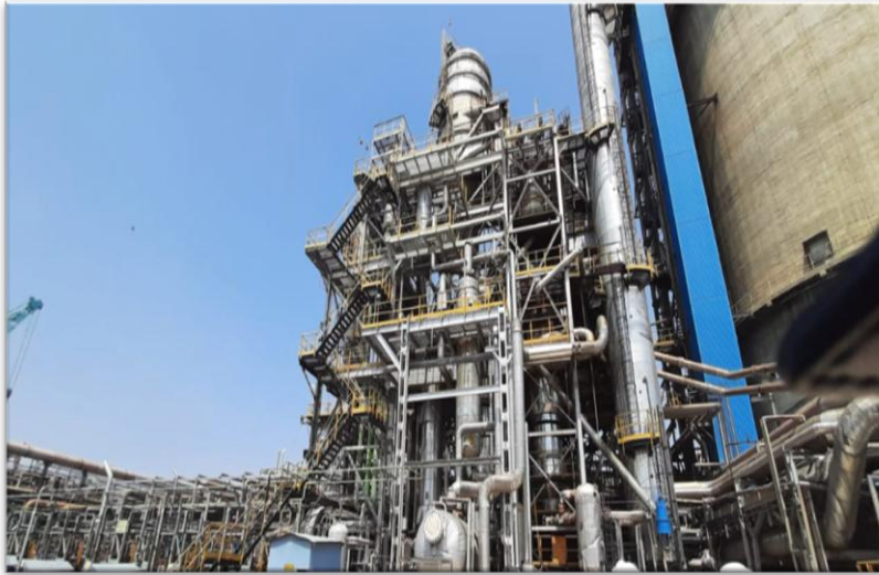
Recovery Unit at the IFFCO Phulpur Unit
