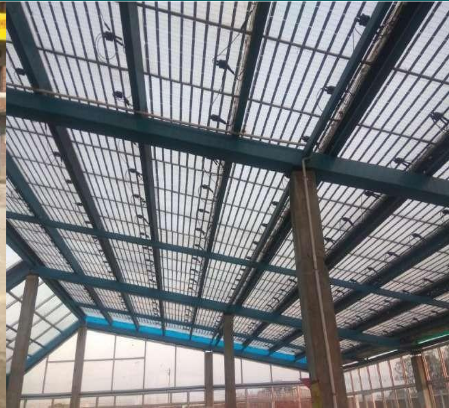
Glass-glass PV module installed at roof of Solar Greenhouse
